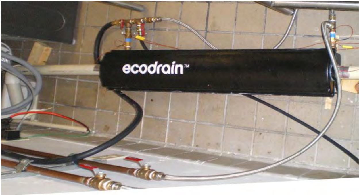
Figure 4: Ecodrain A1000 Setup Behind the Dishwasher
